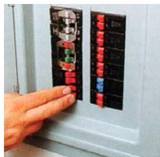
Electricity. Flip off breakers if you find fallen or loose wires or appliance damage, or if you smell burning insulation.
